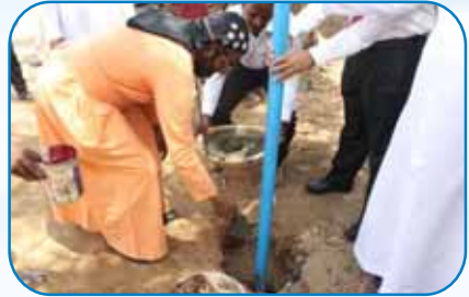
Installation of Playing Area for toddlers at Mar Gregorios Public School, Chennai
